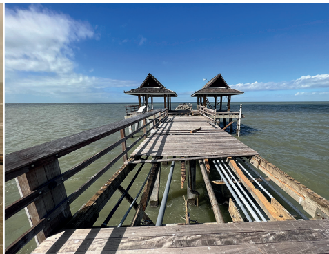
Naples Pier a day after Hurricane Ian
