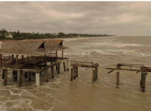
Naples Pier during Hurricane Ian
